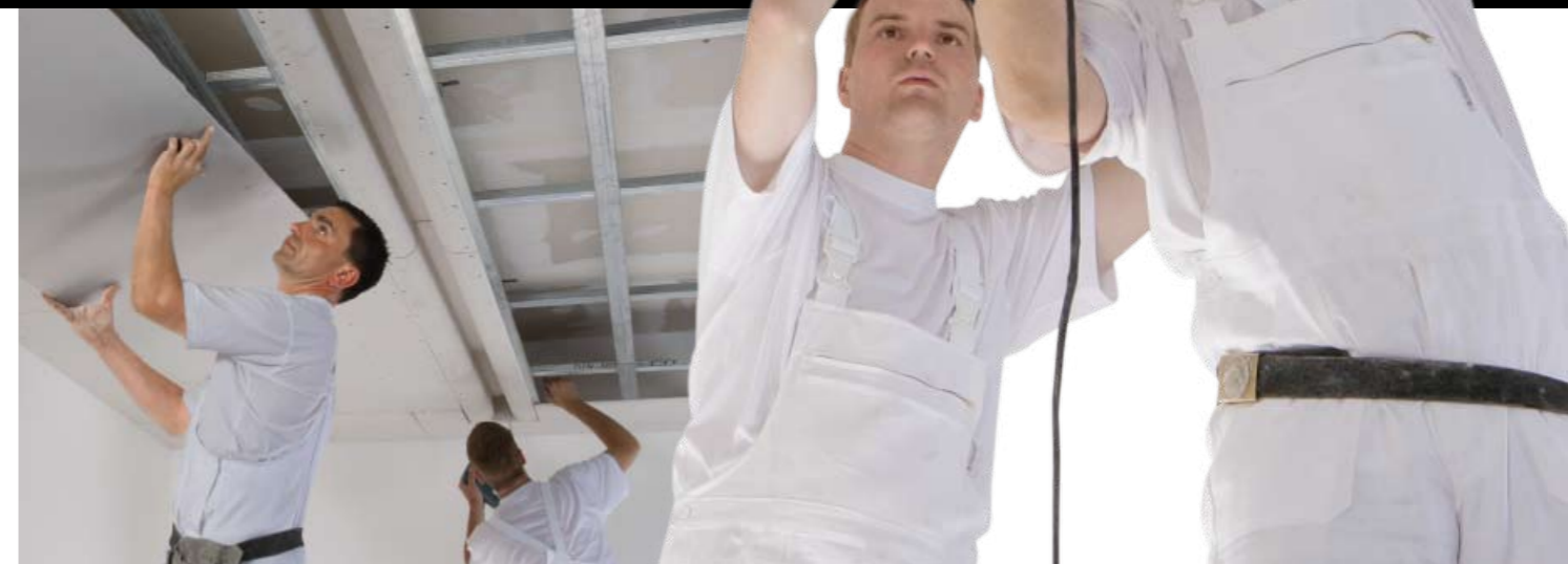
3] The rounded channel contours fit seamlessly into the gypsum plasterboard ceiling.
